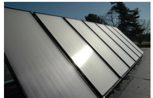
Figure 8 - solar thermal installation on Biddeford Campus Center
