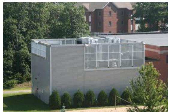
Figure 2 - chiller plant on Biddeford Campus
